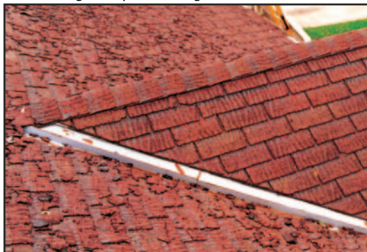
Hail damaged asphalt shingles.
